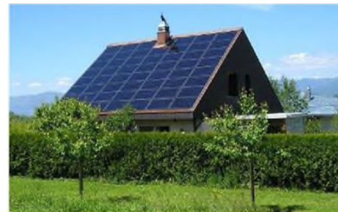
Example of a Solar Conversion System, Structure-mounted
