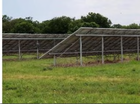
Example of a Solar Conversion System, Ground-mounted
